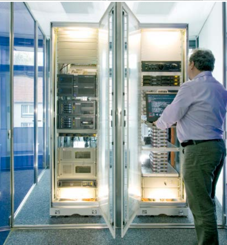
Control room and mainframe of the reservoir control centre of the Ruhrverband in Essen.
