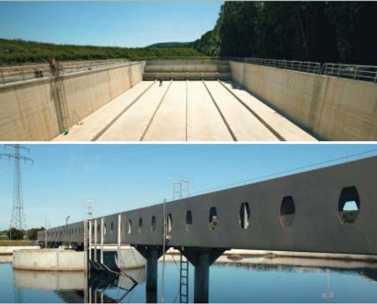
Stormwater tank (above) and sewage treatment plants (below) help to provide clean water.
